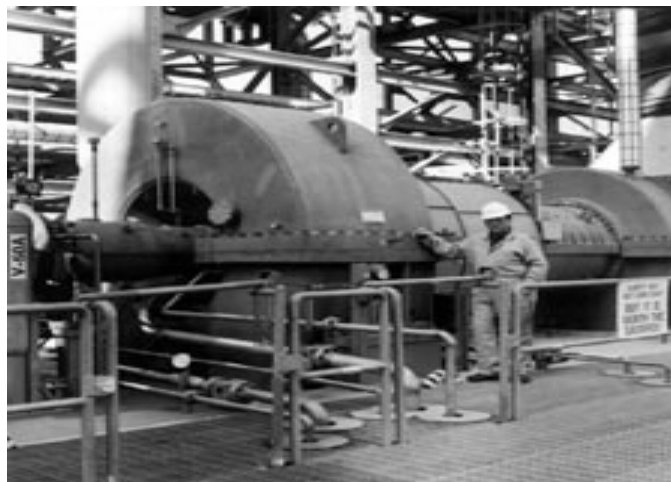
Figure 3 – An Axial-Flow Compressor
