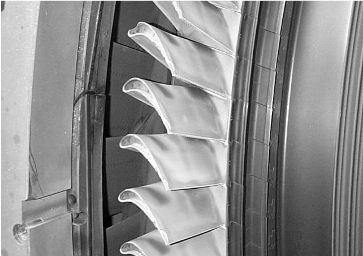
Figure 6 – A Turbine's 1 st Stage Blades
